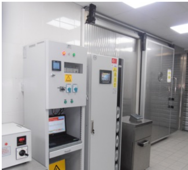
Fig. 6. Test control units and test room for innovative commercial refrigerator prototype.
