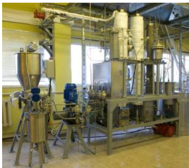
Fig. 8. The view of experimental co-generation power plant CGPP-10 for autonomous energy supply.
