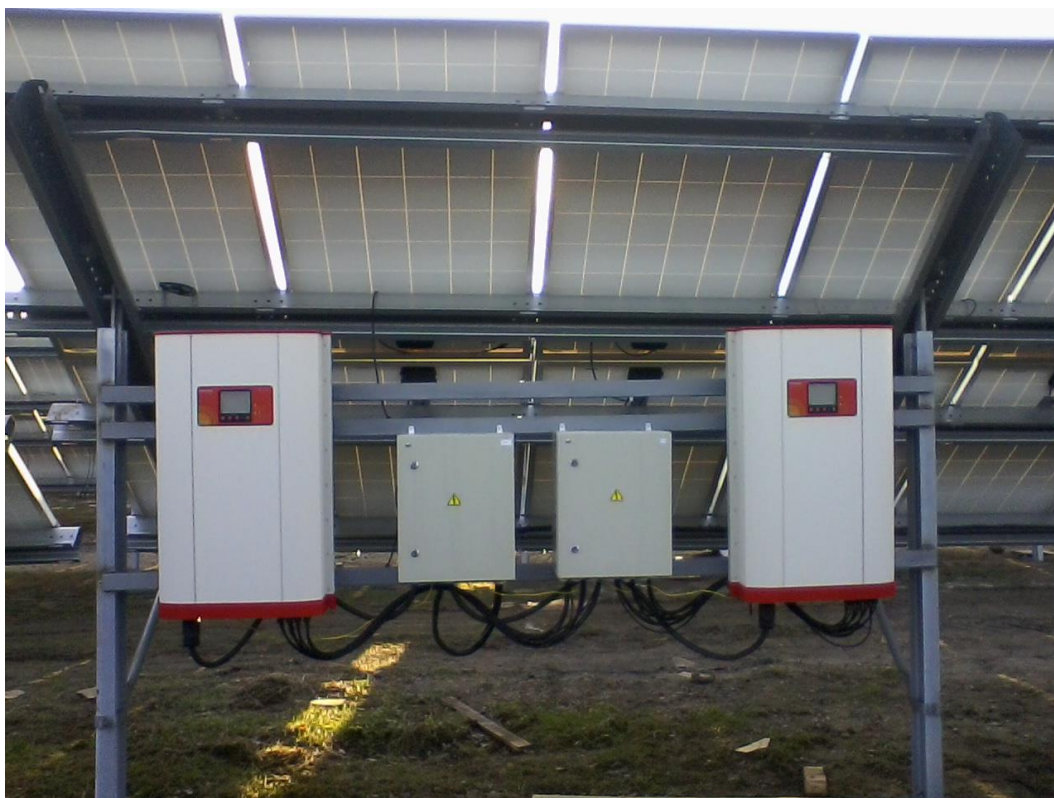
Fig 2. Bobruisk SPP inverters
