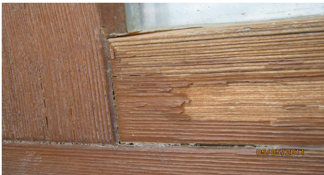
Photo 4. Appearance of coating of horizontal bars of door of sky-bar 9-floor
