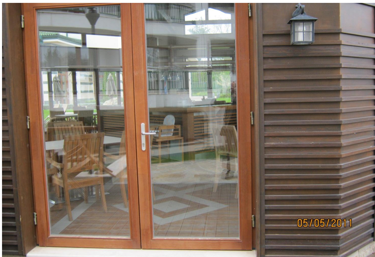
Photo 9. Appearance of coating formed on door bars and siding
