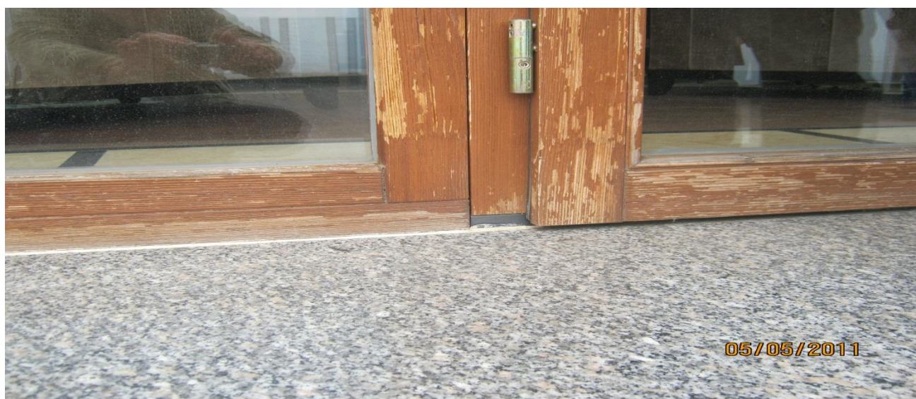
Photo 2 . Appearance of door coating of sky-bar 9-floor
