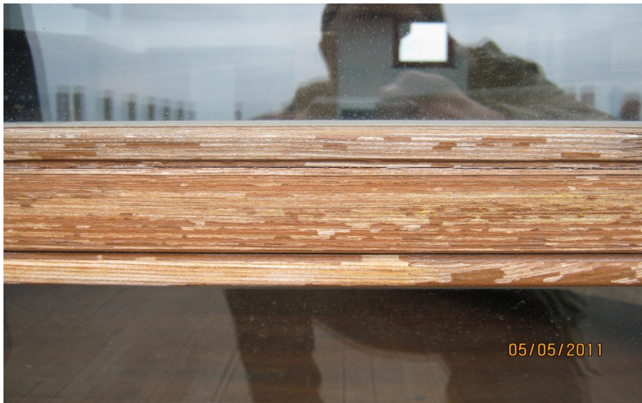
Photo 3. Appearance of coating formed on horizontal door bars of sky-bar 9-floor
