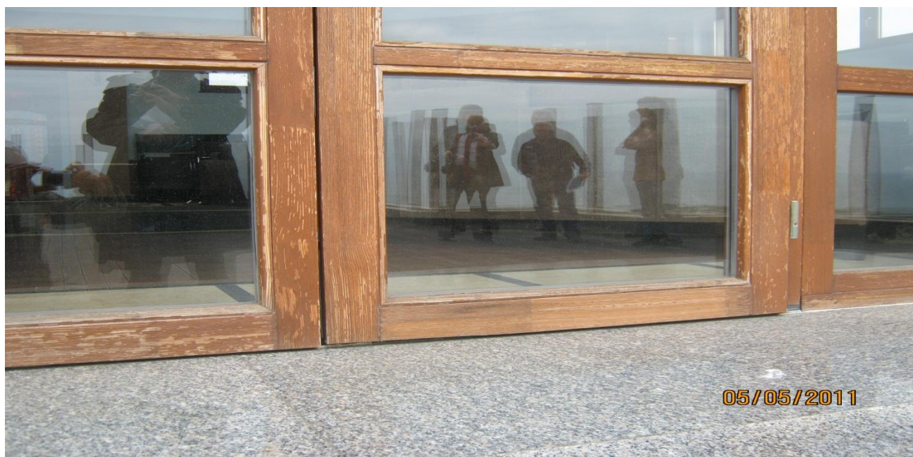
Photo 1 . Appearance of door coating of sky-bar 9-floor
