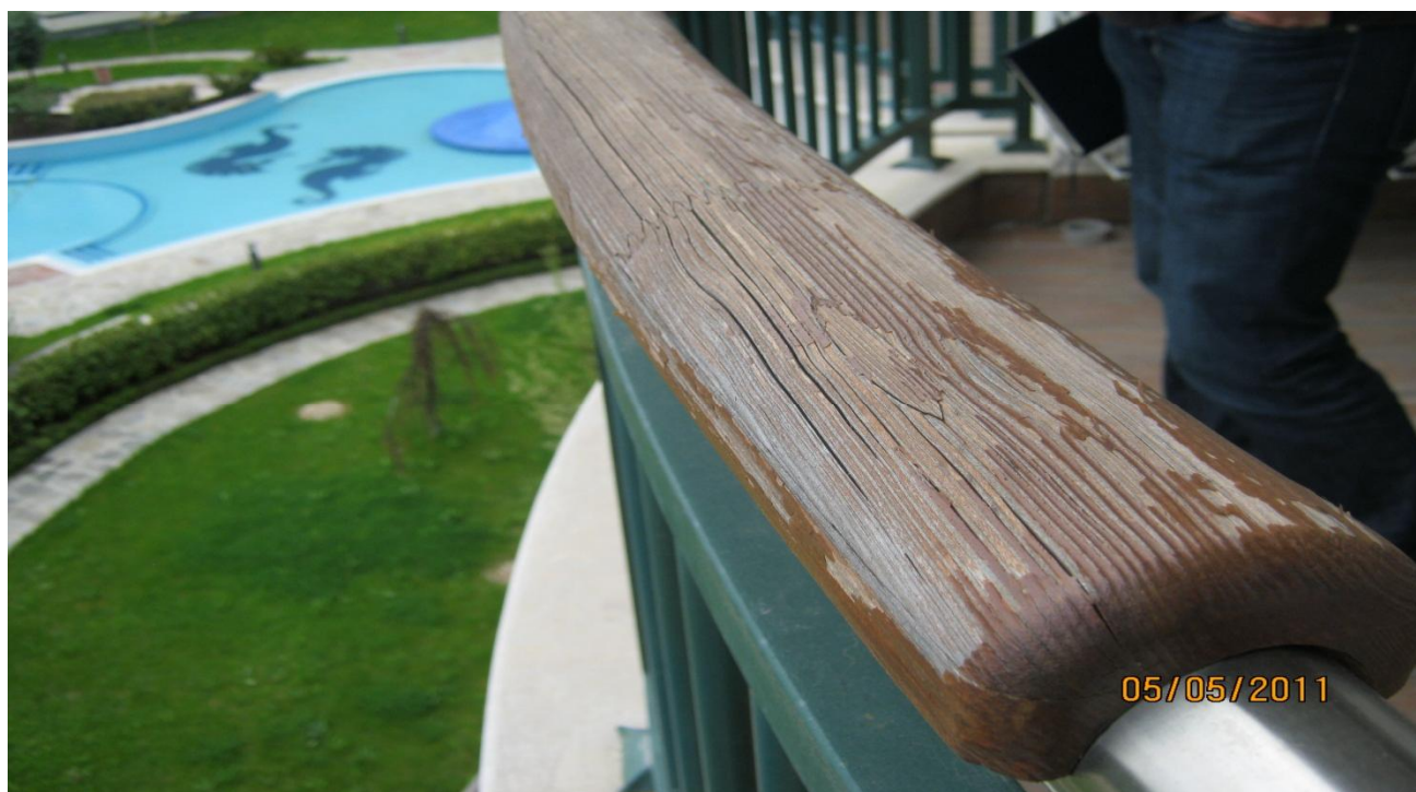
Photo 5 . Appearance of coating formed on rustic parapet handles
